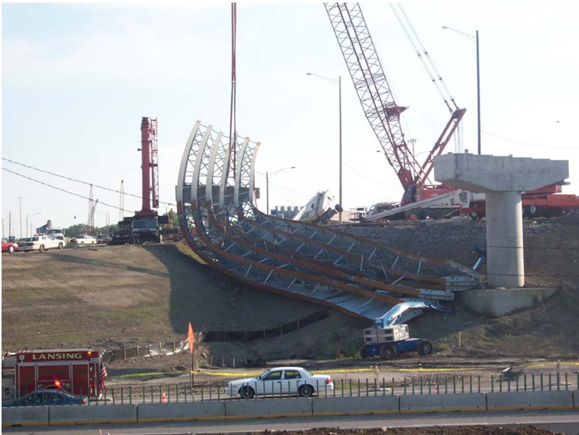
Figure 1.3: Illinois I-girder Bridge Collapse during Construction (Photo Courtesy of ILDOT)
