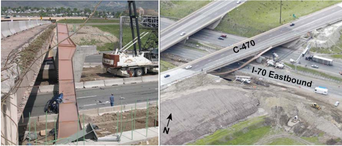
(a) Buckled I-girder
